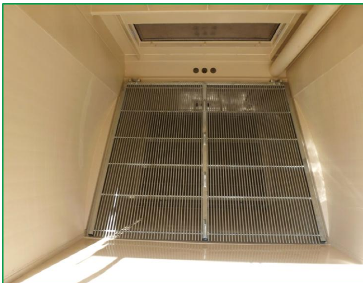
Internal view with the screening grids in position
